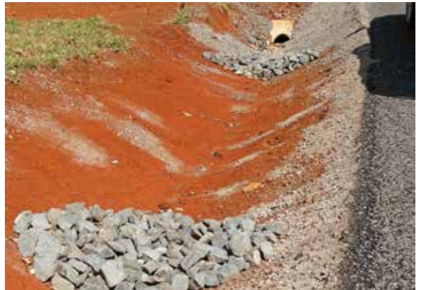
Combatting sediment runoff: sediment control devices installed in a steep roadside drain by council staff
