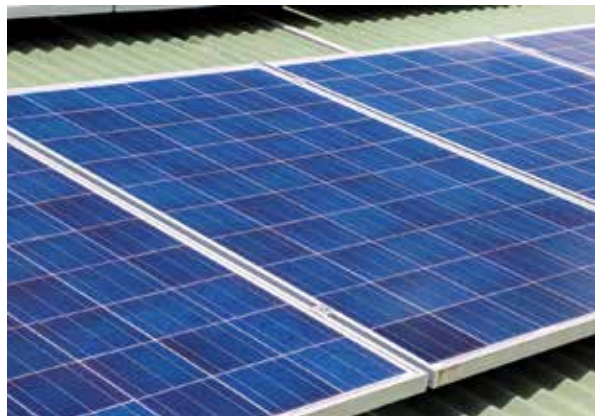
Storing power: rooftop solar panels at the SES building in Diwan
