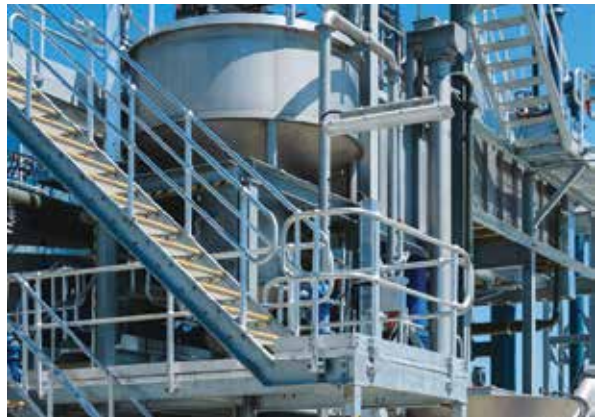
In with the new: Sarina now has a state-of-the-art water recycling facility
