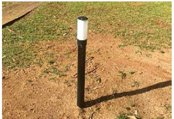
Energy efficient LED bollards placed in public areas.
