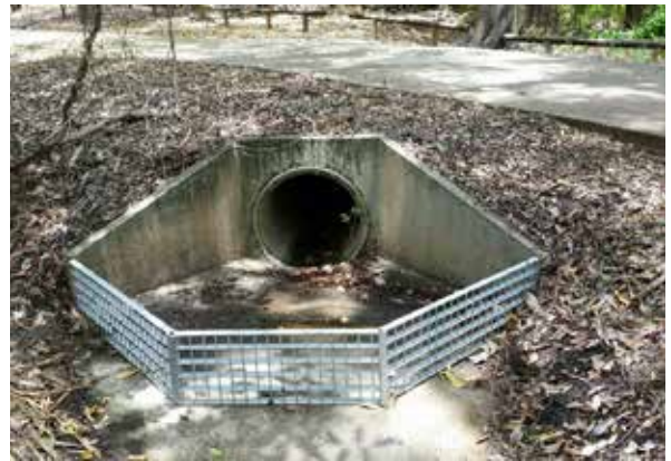
Trapping trash: a pollutant trap installed at Baldwin Swamp Environmental Park
