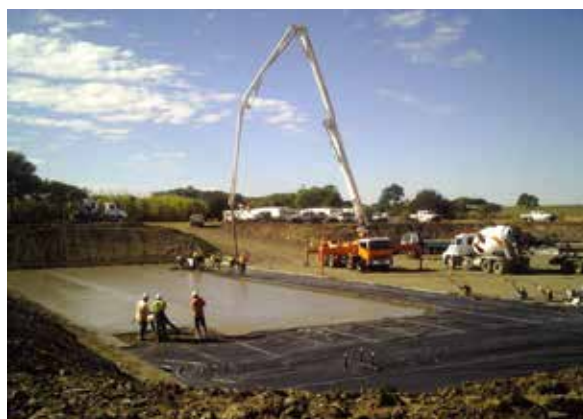
Construction underway: installation of the digester blinder slab at the Rubyanna Wastewater Plant
