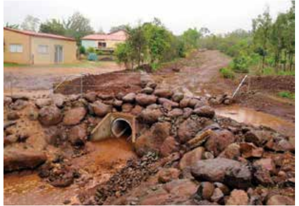
Stormwater slowdown: drain constructed at Hutton Drive, Rangeview, using watershed restoration techniques
