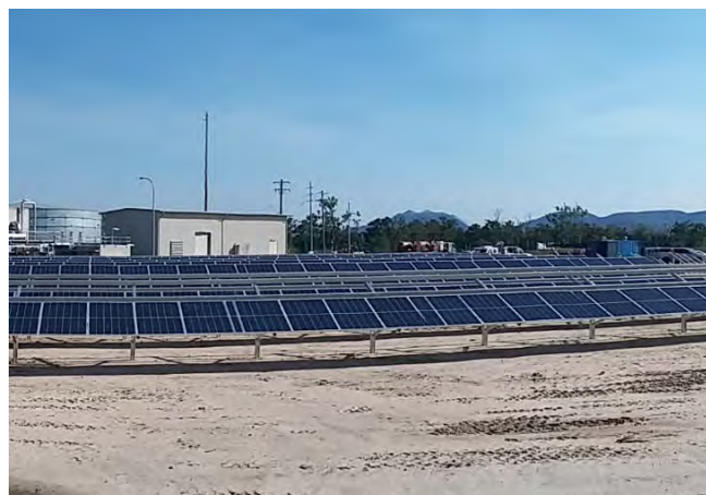
Bowen Water Treatment Plant – solar array
