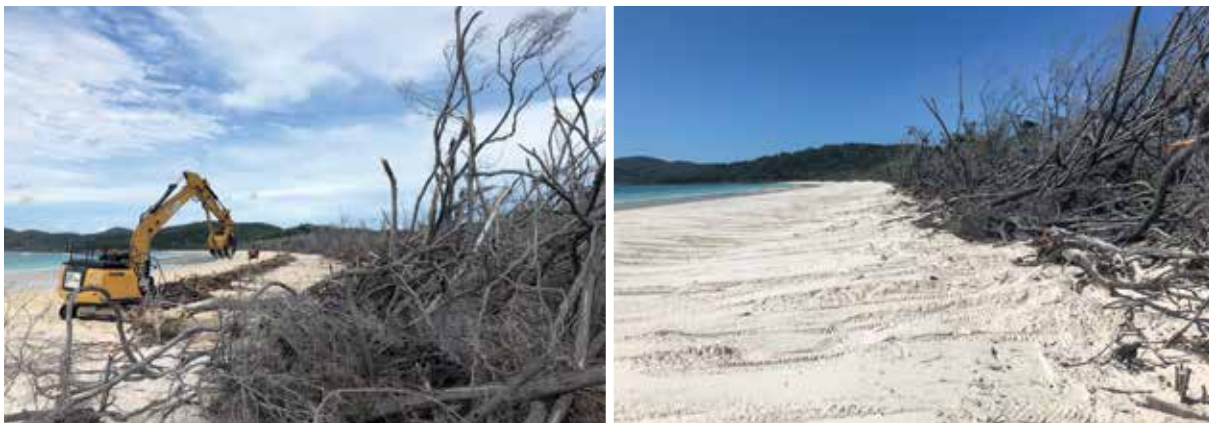
Figure 4.2 Cyclone damage on Whitehaven Beach, 2017 Whitehaven Beach in the Whitsundays is renowned for its long white sandy beach. Left: Post-cyclone clean-up. Right: Re-profiled beach. © Queensland Parks and Wildlife Service 2017
