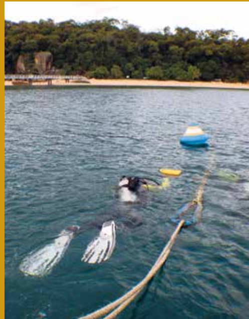
Rangers inspecting newly installed moorings at Yanks Jetty, Orpheus Island. © Queensland Parks and Wildlife Service 2019
