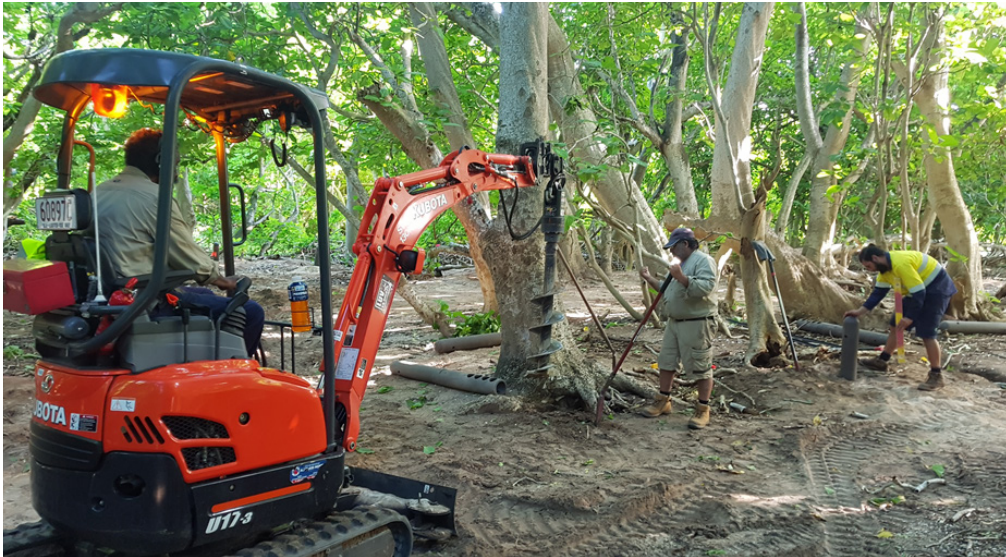
Construction of boardwalk at North West Island as part of the Reef Joint Field Management Program © State of Queensland (QPWS)
