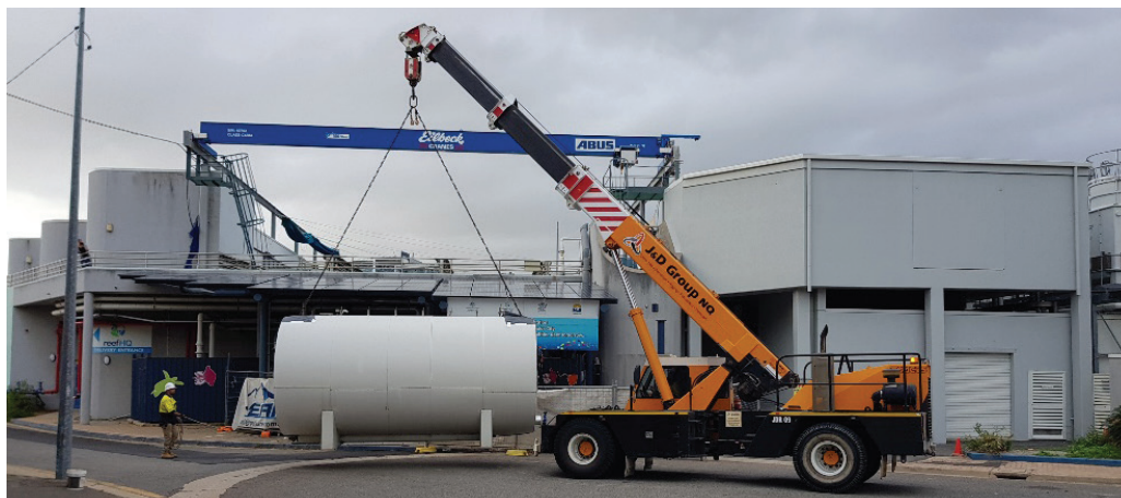
A storage tank for chilled water was removed to enable construction of Reef HQ Aquarium's new access facilities. © Commonwealth of Australia (GBRMPA), Photographer: Jo Hurford
