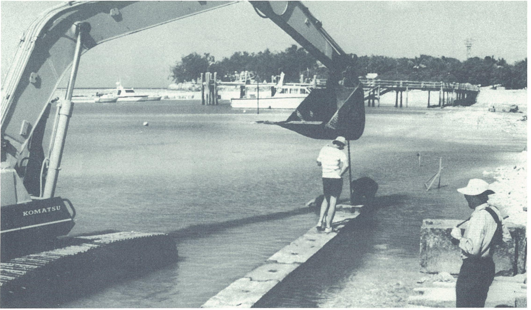
Engineers from the Queensland Department of Environment and Heritage on-site during construction of a bund wall at Heron Island harbour.
