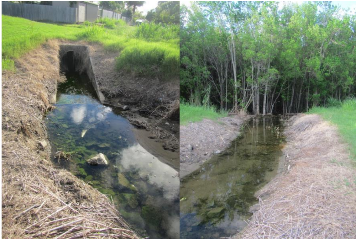
Figure 2.5.5: One of many stormwater drains in urban areas that flow directly into adjacent mangroves
