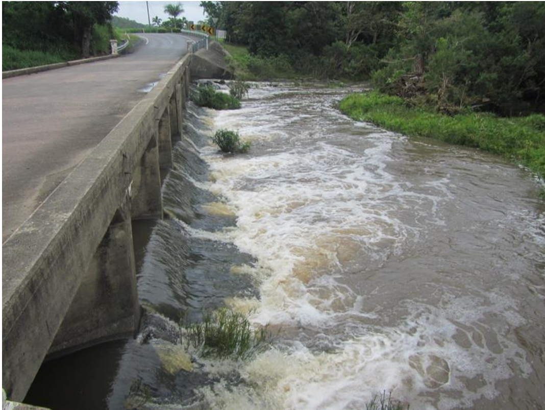
Figure 2.5.4: Reliance Creek sub basin – road crossing with fish ladder and fish friendly design
