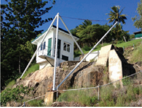
Dent Island winch house and derrick crane after restoration works. Photograph courtesy of Queensland Parks and Wildlife Service.
