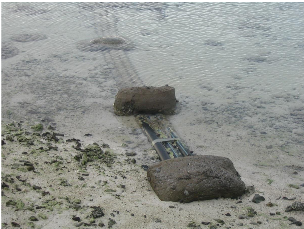
Figure 14. Water intake pipe ( source: GBRMPA )
