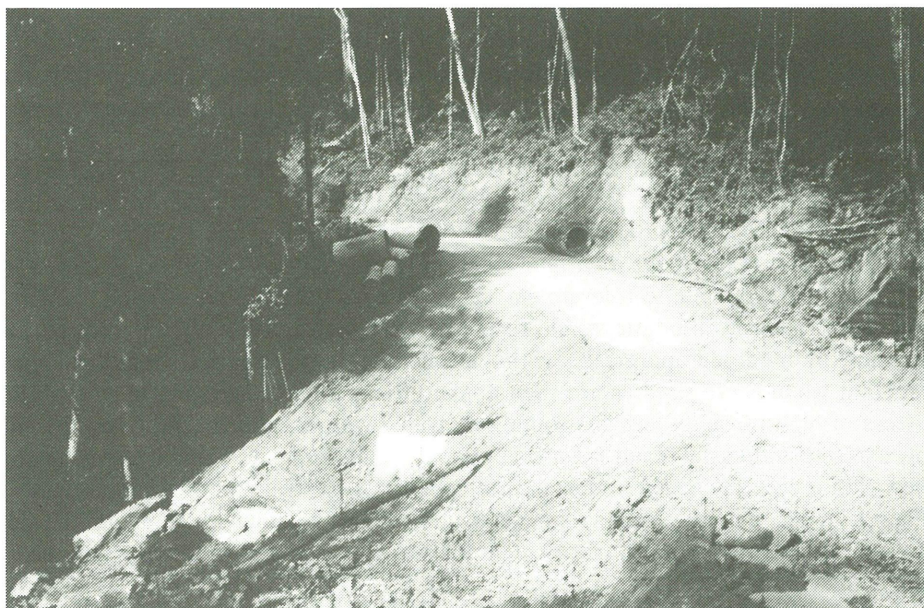
FIGURE 18. Gullying and landslips are frequent after heavy rain especially on steeper road sections. Potential remains for complete slope failure and massive sediment yield.
