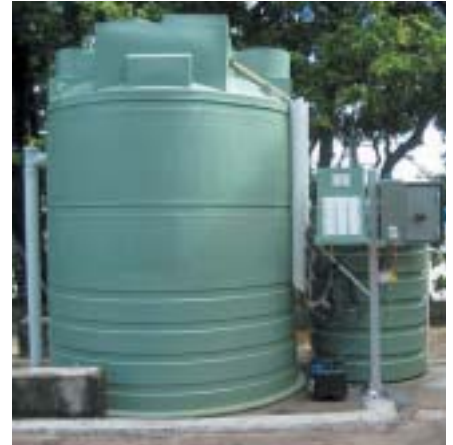
The new tertiary water treatment plant at Low Isles is exceeding expectations
